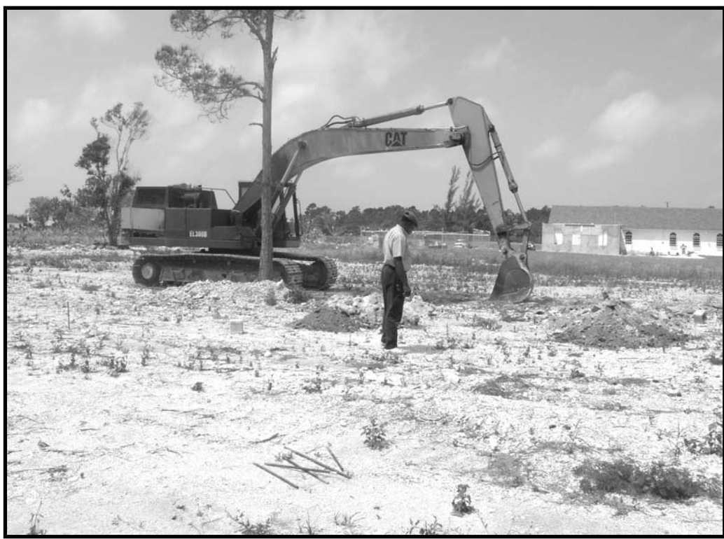
Work began on the new Bahamas Academy of Seventh-day Adventists this week at the Marshall Road site. In the photo above is Howard Barr, is watching as the trench is being cut.
