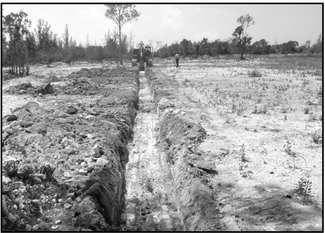
The Bahamas Academy Secondary Division foundation is on its way. On Tuesday, April 26, 2005, workmen began cutting the footing for the multi-million dollar new complex for Adventist education in Nassau.
